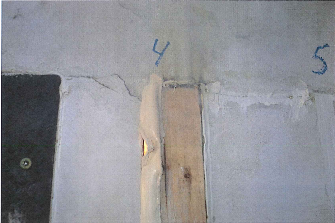
Photo No. 9 Integrity failure at the top of joint seal 4 after 90 minutes of testing
